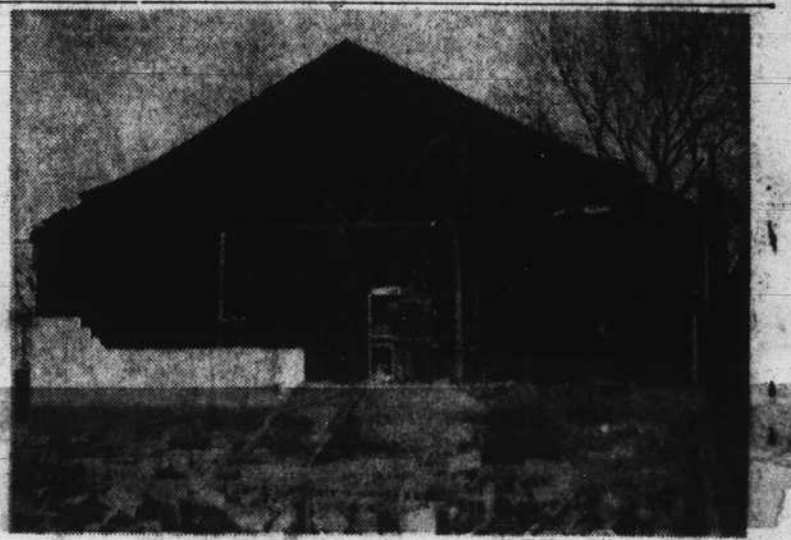
BIG WIND FROM SOMEWHERE—Last Friday afternoon's wind and rain storm did spasmodic damage throughout the area. Most spectacular, probably, was to this building at West Hillsboro, a block-front storage warehouse next door to the Hillsboro Savings & Loan office. A quick gust of wind knocked off the complete front, as the picture shows, and sent blocks sailing all the way across the street.
