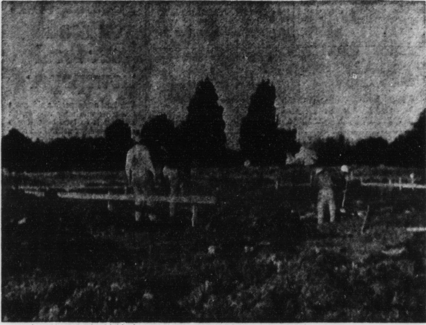
NEW PRESBYTERIAN CHURCH UNDERWAY —A. L. Jarrell & Sons of Salisbury have under construction the North Hills Presbyterian Church, located on Highway 601, between Franklin and Catawba College. Plans for completion are in early June of this year.
