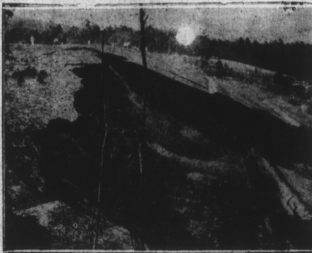
This photo shows water gradually trickling from the great dam at Greenville, S. C. which suddenly cracked causing thousands of persons in the Saluda Valley to flee their home.
