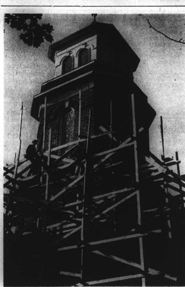
STEEPLE GETS PAINT—The clean-up campaign in Mount Olive officially ended nearly two months ago, but that hasn't stopped the town folks from making improvements on their property. An example of Mount Olive's continued interest in a clean city is shown in the above photo as workmen prepare to paint the steeple at the Presbyterian church.—Staff photo by Vaden Brock.
