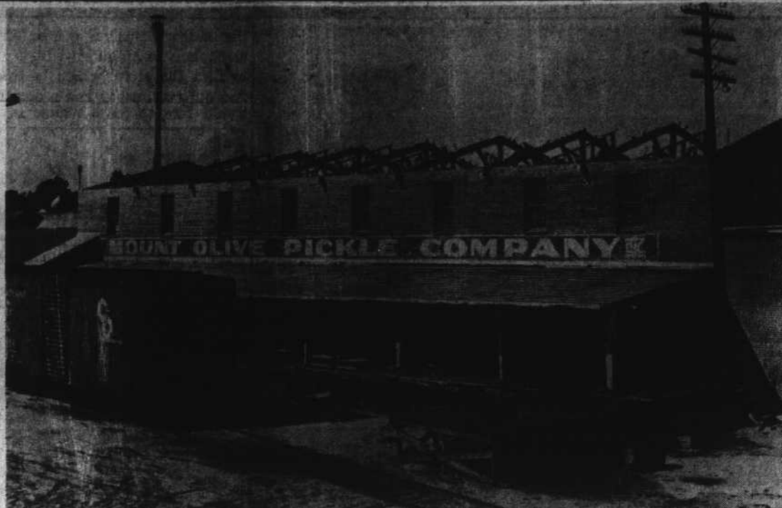
ROOFLESS —This is what Hurricane Hazel, which struck in this area Friday, did to the roof of a storage house belonging to the Mount Olive Pickle Company. It took the roof, intact, and blew it out across the railroad tracks.—Staff Photo by Vaden Brock.
