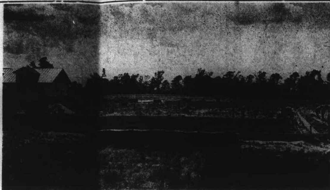
MORE CLASSROOMS — A combination classroom-gymnasium goes up at Carver school. One of three buildings now being erected on the school campus, it is expected to be completed later this year.—Staff Photo by Vaden Brock.
