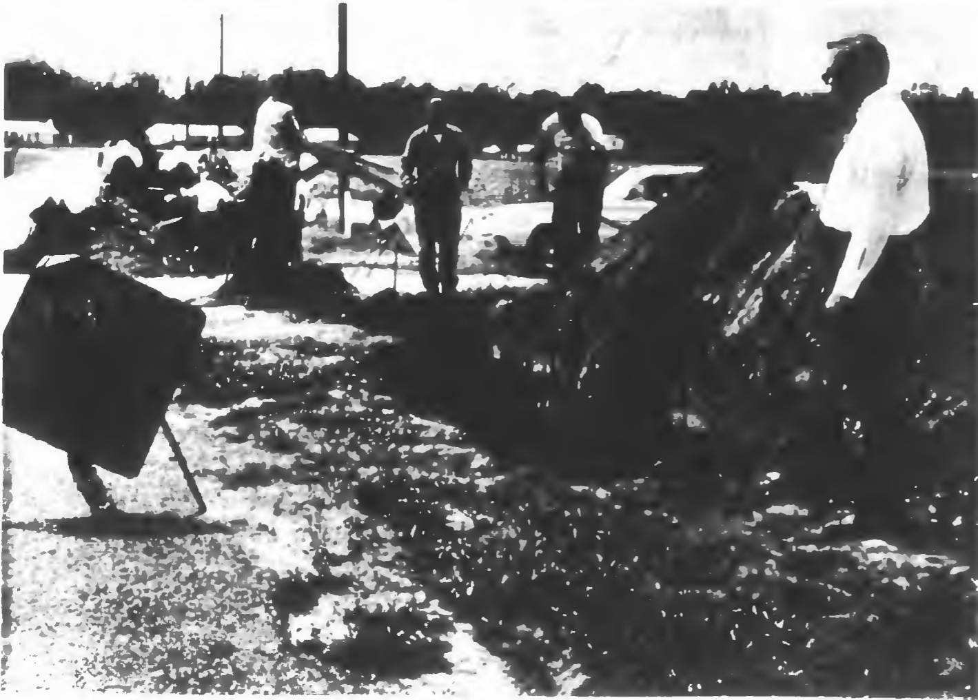
FOR SUNSET HILLS -- The Town of Raeford had to hire a Charlotte firm to come and bore beneath the highway in order to comply with regulations in installing a new water line to the Sunset Hills section. Some 1,300 feet of new six-
