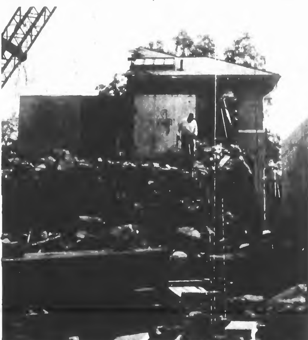
JAILBREAK -- Many aviator of the law wishes this had happened while he was incarcerated in Hoke County Jail. The old jail is being torn down, while a new one is being raised nearby. The box-like steel structure behind the worker on the rubble is the second floor cell block. Hoke's prisoners are being housed in the Scotland County jail at Burlington while the new Hoke jail is being completed.
