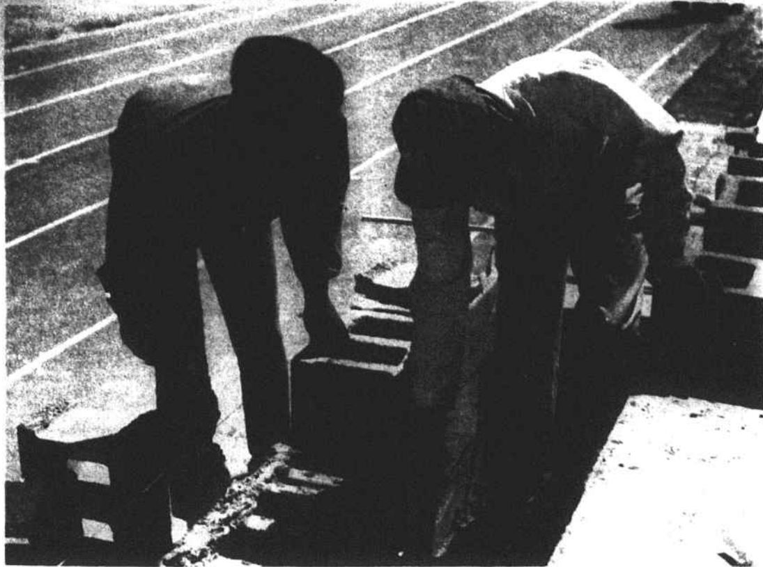
LAYING BLOCKS -- Weldon Graham and Lendward Simpson, instructor, lay concrete blocks along the track at the stadium.
