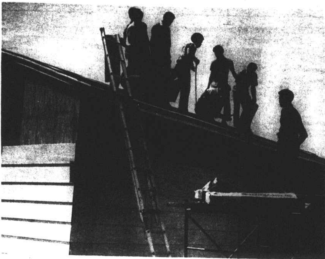
ROOFING - Vocational education students nail shingles at one of the portable classrooms under construction at the high school. The buildings were designed and built by Hoke vocational students under the supervision of their instructors with funds provided by the Emergency School Act this fall.
