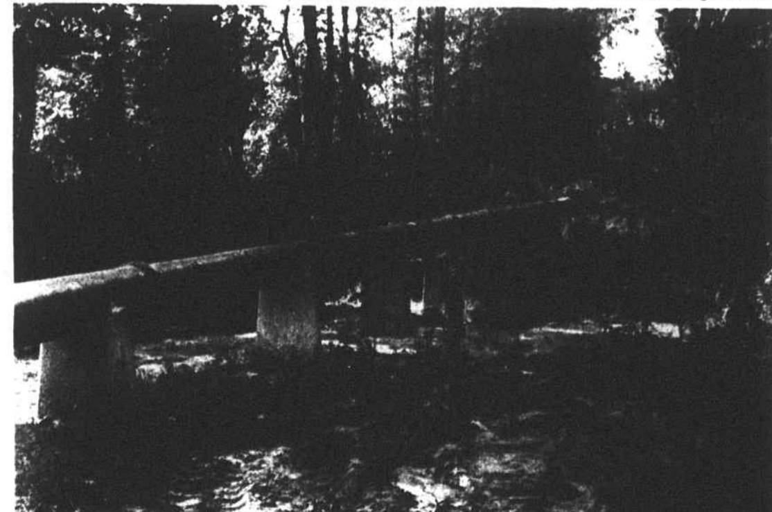
LAST MINUTE ADJUSTMENTS - Roy Davis and Joe Bellas make some final position changes in the new sewer line that will connect Kilt-Away with the city system. The line was inspected and put into operation Tuesday, ending the need for the city's makeshift irrigation pipe system that has pumped wastes from the textile plant for the past ten months.
