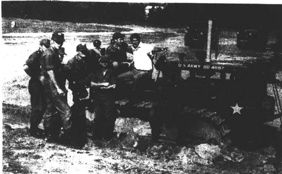
UPCHURCH LANDSCAPING - Members of an engineer battalion from Ft. Bragg pause to get directions from W.K. Morgan, assistant principal at Upchurch School. The playground has been graded and gullies have been filled in to provide space for another basketball court, other play areas and a picnic area for community use, through an Army-aided program to help increase recreation facilities in that area. Shown here are (from left) PFC Joseph Deering, SPS Ray Morrisette, PFC Thomas L. Jones, 1LT. Charles K. Morrison, SPS Bruce Keener, SPS William Gogson, dozer operator, Morgan, and PFC Fred Clinton. They are members of HHC, 307th Engr. Bn., 82d Airborne Division.
