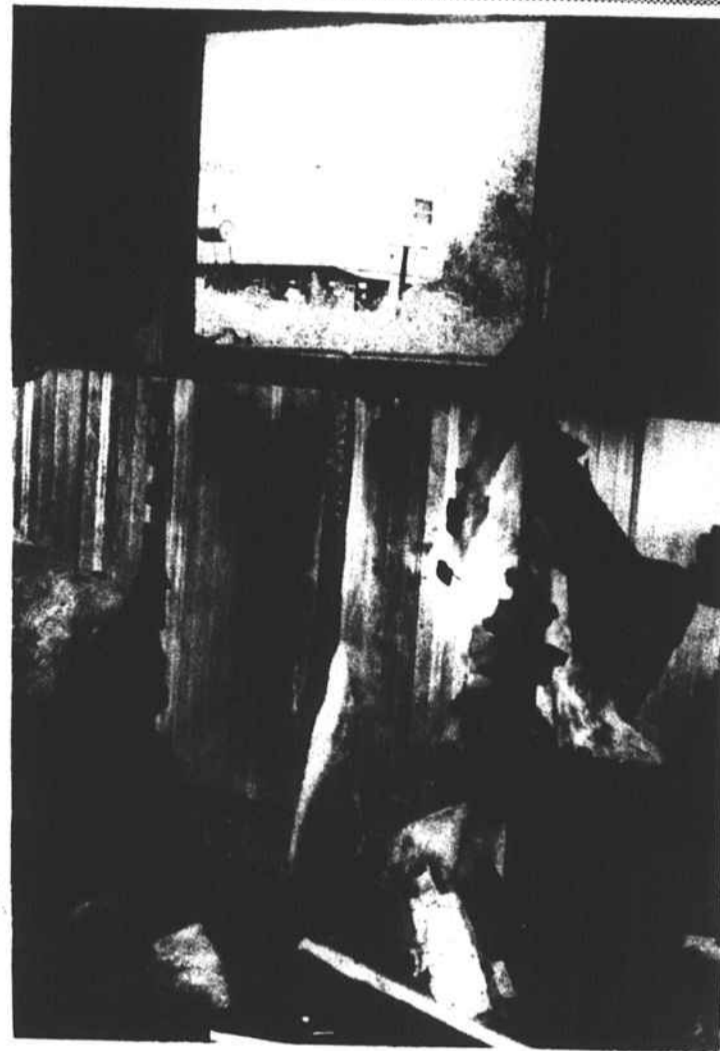
FIRE DAMAGE - Interior of the burned out trailer belonging to Betty Young, of the Oakwood Trailer Park. Authorities suspect arson as the cause of the Monday night blaze which caused $2,500 damages.
