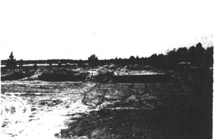
WORK BEGINS - Site of new board of education building shows construction changes as work begins on Woolley Street land south of Harris Ave. Chisholm Construction Co., Rockingham are general contractors for the $185,935 building. Their low bid on the project was $107,360. Hayes-Howell and Associates are architects for the project. Completion time for the building was set at 240 days. (N-J Photo)
