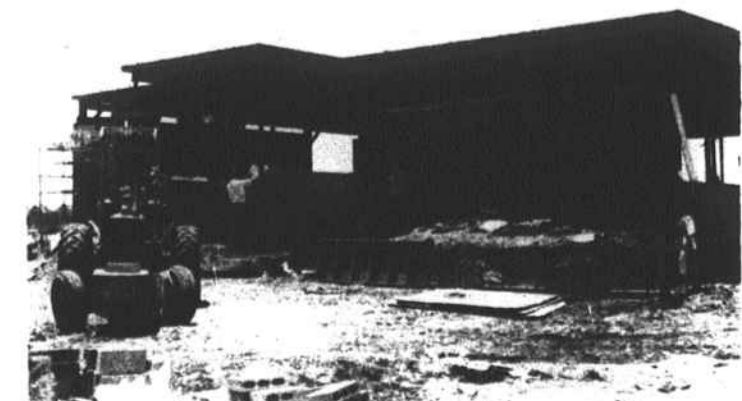
NEW BUILDING - Construction on new Board of Education Building on Wooley Street progresses. The structure is being built by Chisholm Construction Co., of Rockingham, on 4.43 acre tract on west side of Wooley Street south of Harris Ave. The Board of Education land purchased from Robert and Mamie Gatlin includes a 9.95 acre tract on east side of Wooley for a total acreage of 14.38. (N-J Photo)
