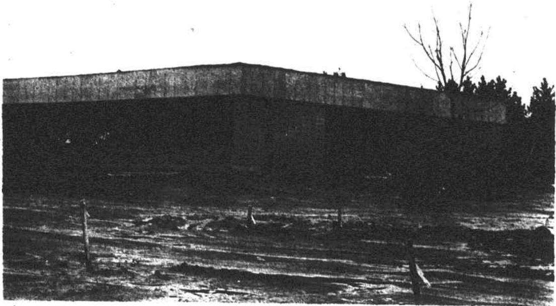
TAKING SHAPE — Work on the new county office building under construction on Magnolia Street is progressing in spite of the recent rain which has left a field of mud for the setting.
