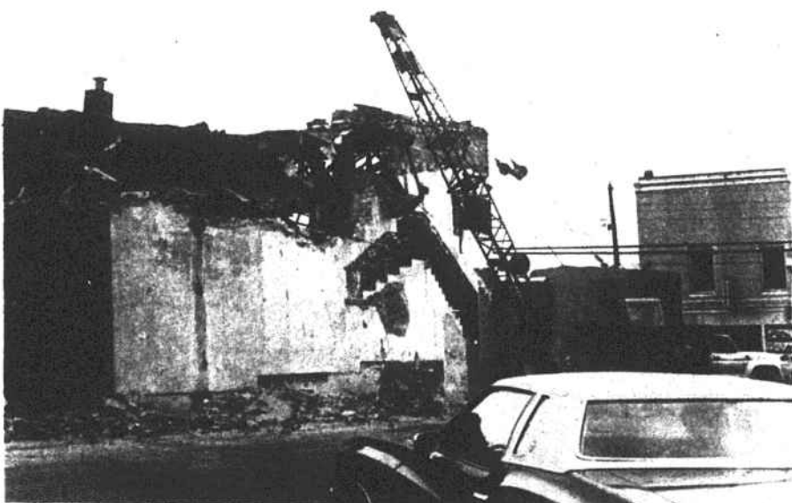
BOOM! POW! -- The look along Main Street is changed in April with the demolition of the old theatre building.
