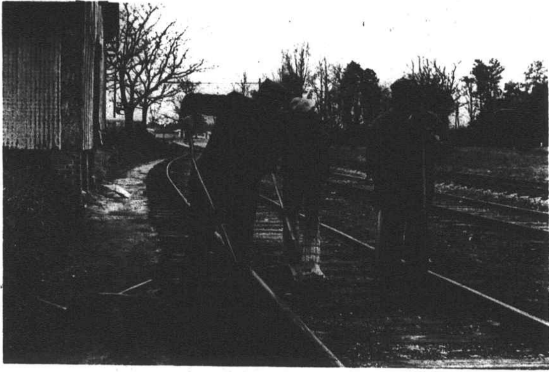
WORKING ON THE RAILROAD - Aberdeen and Rockfish employees put the track in order Monday. They also began work to smooth the railroad crossings in the city.
