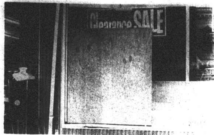
UNEXPECTED INTRUSION - A car crashed into the front of the Super Dollar Store on South Main early Saturday morning, breaking the glass.
