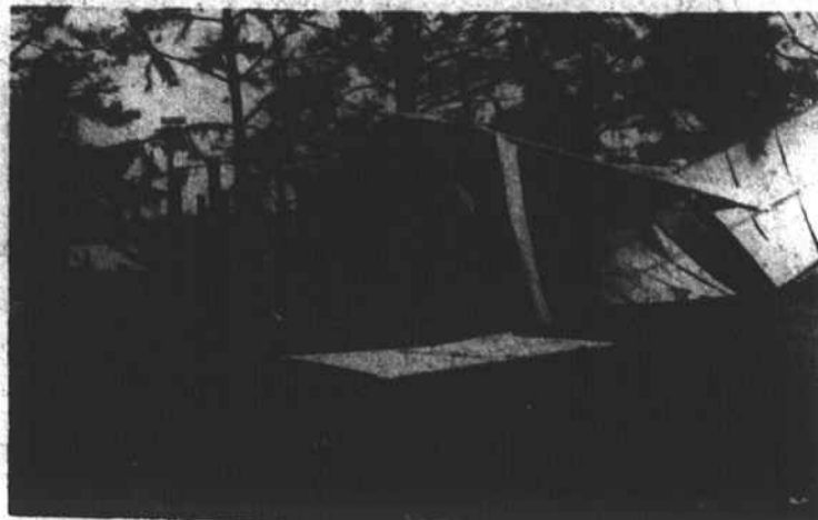
CAVED IN - June Wright's metal storage shed was blown across the yard by a storm early Friday morning. The shed was anchored by concrete blocks, one of which can be seen in the foreground.
