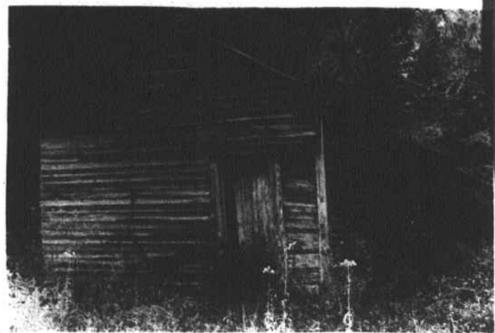
PINE FOREST...Abandoned in the 1920's, the building still stands on U.S. 401 near the county line.
