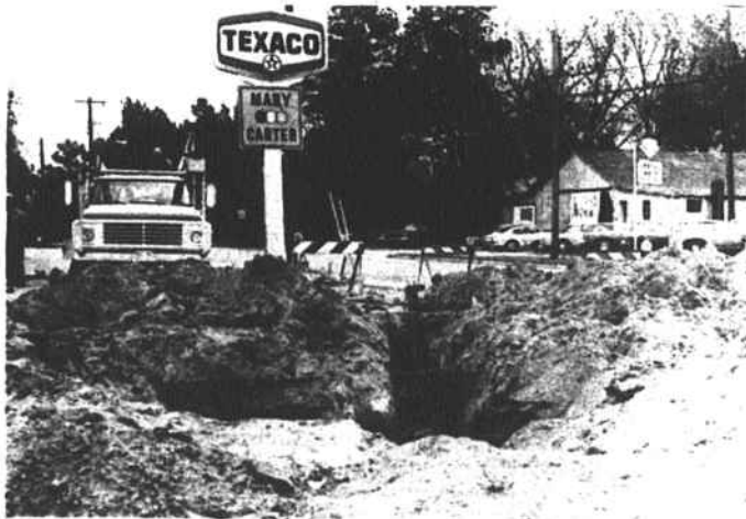
DIGGING- Bethel Rd. north of Harris Ave. was closed while workers dug away to put in sewer pipes. The street is slated for curbs and gutters.
