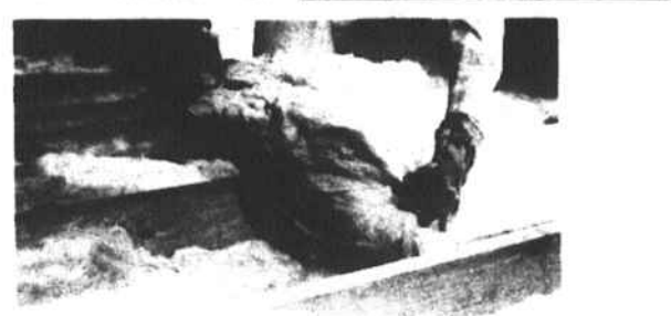
1-2-3 -- Insulating your attic and realizing savings on heating and cooling costs is as easy as one, two, three. Start with a sharp knife and a straight edge to cut into the proper lengths.
