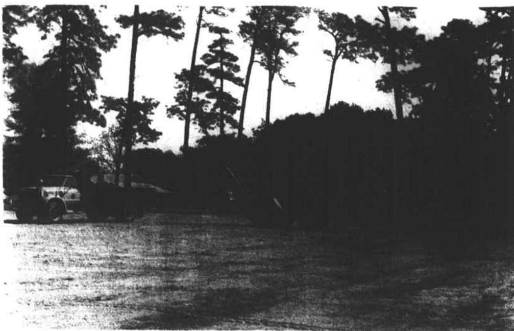
CONSTRUCTION—Work has begun on three tennis courts in the McLaughlin playground area, which are expected to be ready by summer. Costs of the new courts is being paid out of this year's recreation commission budget.
