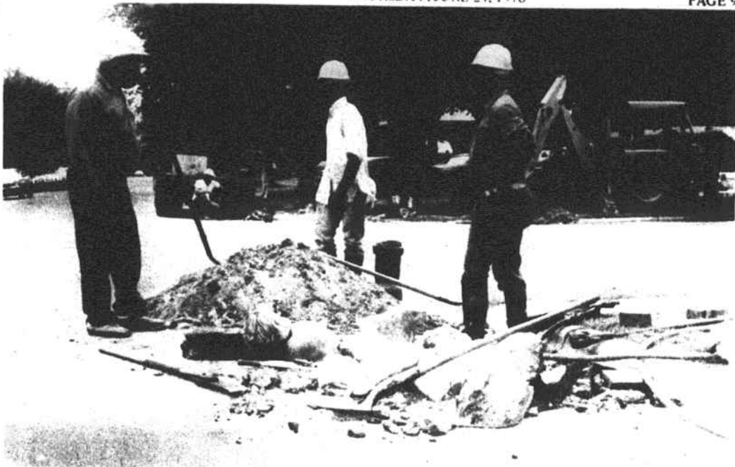
REPAIR—City water was shut off to a portion of the downtown area for two hours Monday morning while repair crews worked at the Magnolia St. and W. Edinborough Ave. intersection. A hit and run driver knocked down the fire hydrant in front of the Presbyterian Church over the weekend.
