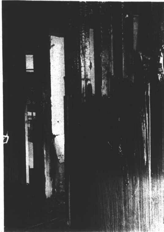
FIRE DAMAGE —Fire damaged a home in the Scurlock School area late Monday night. Hillcrest Volunteer Fire Department responded and saved all but two rooms of the house. The family was not at home at the time and no injuries were reported.
