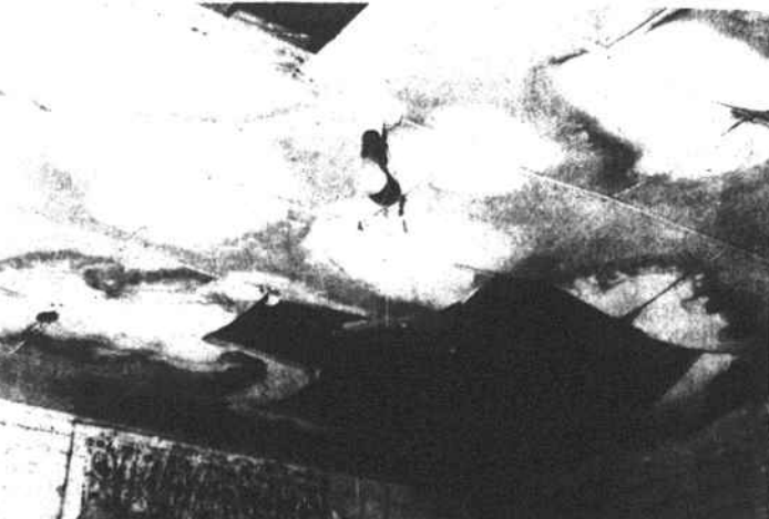
KITCHEN CEILING -- The unsightly and dangerous ceiling here will be repaired at no cost to the elderly homeowner, thanks to one of the housing assistance programs operated by the Robeson County Church and Community Center. Besides improving the appearance, the repair will greatly bolster insulation, often a problem with substandard homes.
