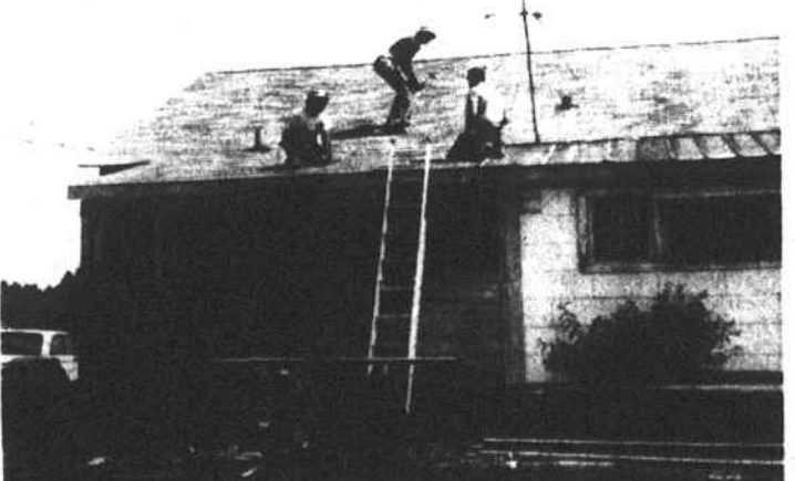
HOUSE REPAIR -- James Billinger, contractor, and helpers James Hammond and Lorenzo Murchison, are at work finishing the new roof at Mrs. Maggie Brown's residence near South Hoke. The work was made possible through a grant received by the Robeson County Church and Community Center, Inc.
