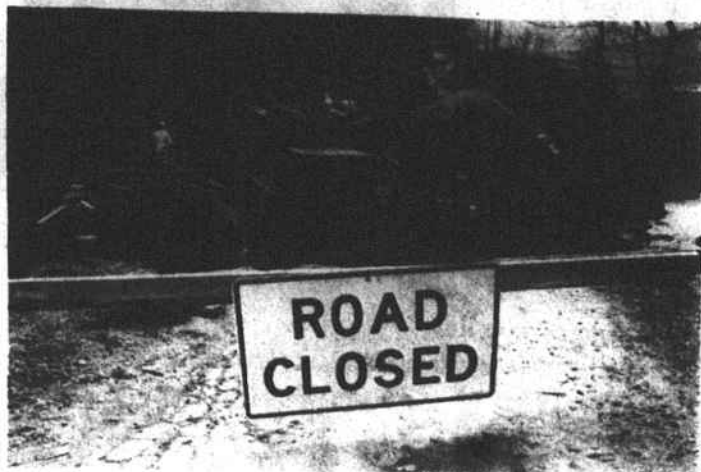
WASHED OUT -- Over 390 miles of roadway in the North Carolina mountains was damaged by floods early in November. So many roads were damaged that the State doesn't have enough signs to mark them all. Department of Transportation crews are working overtime to repair damage in the 16-county disaster area.
