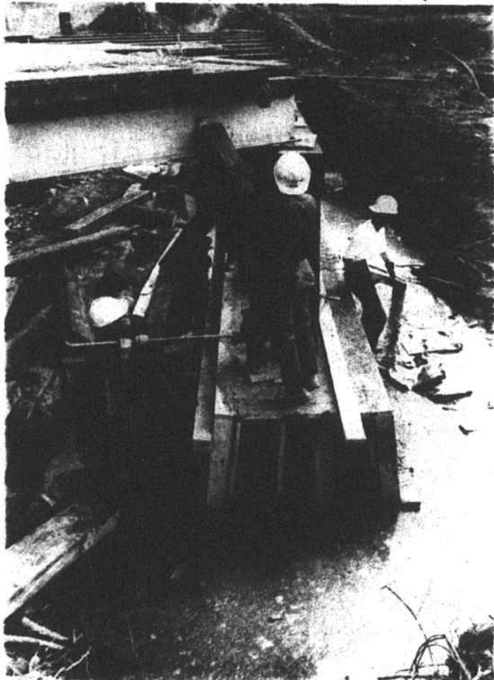
REPAIR BRIDGE -- A DOT maintenance crew struggles to replace the washed-out span on the bridge over Turkey Creek just north of Leicester in Buncombe County.
