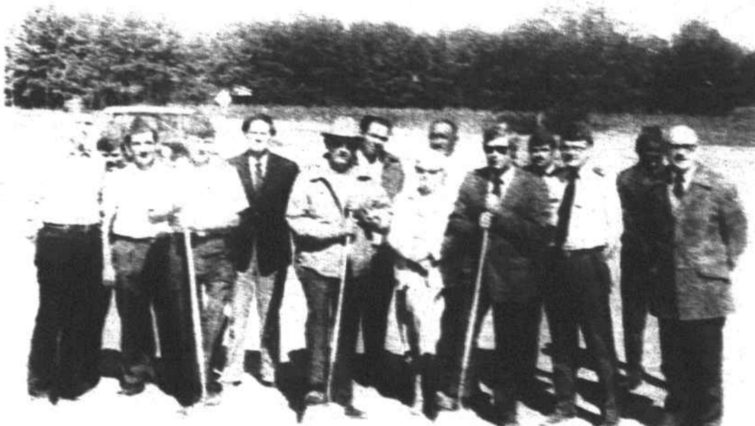
GROUND BROKEN -- At the ground-breaking ceremony for the new National Guard Armory were, front, with shovels, L-R, CW 3 Jesse Jones of Raeford, Raeford Mayor Pro Team Graham Clark, and John Balfour, chairman of the board of Hoke County Commissioners. The others are, L-R, Maj. George Paris, commander of the Guard's Second Battalion, 252nd Armor, SFC Richard Wolf of Raeford; SSG Frank Brown of Lumberton; Earl Fowler, executive vice president of the Raeford-Hoke County Chamber of Commerce; County Commissioners James A. Hunt, Mabel Riley and Neill McPhatter; MSG Charles Hurvill; Lt. Col. Elbert McPhaul, Jr., director of facilities, State Crime Control and Public Safety Department; Sgt. Cooper, and Gilbert M. Slack of White and Slack, Raleigh architect firm which designed the building. [Staff photo by Pam Foderick.]
