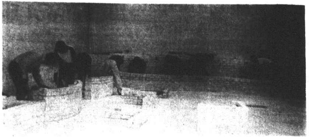
GARDEN WALL COMING -- These students of Lendward Simpson at Hoke County High School are building a decorative garden wall in their masonry class. Simpson said it's a complicated job because there are no straight lines in it. The students in the photo are Christopher Cameron, Julia McNealey, James Douglas, Sarah Morris, Brendick Washington, Arletha Williams, Bernice McMillan, Ronnie Malloy and Richard Brewer.
