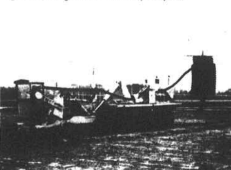
Laser operated drain tile machine can install 100 ft. of tile per minute. This past March, this machine alone installed 131,276 ft. on Hoke County farms.
