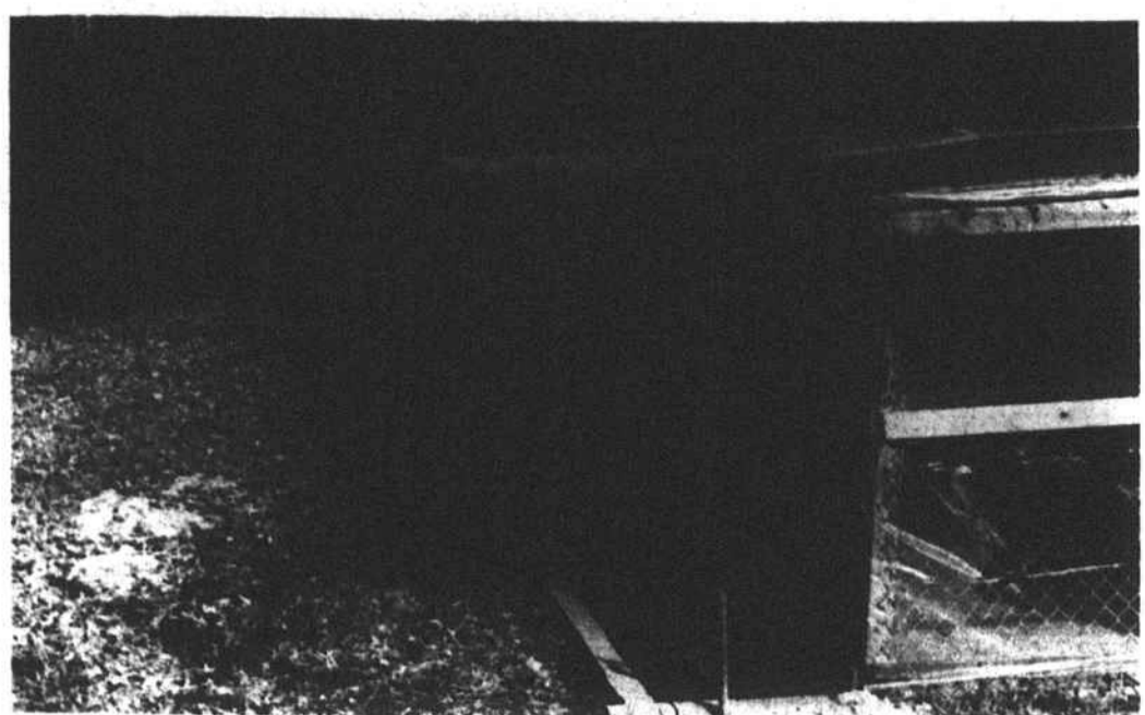
FOR WARMER ANIMALS -- The rear side of the pens at the Hoke County dog pound is sporting newly installed vinyl sheeting to protect the dogs and cats from the winter wind, making living considerably warmer. The concrete trough outside the bottom of the pens was installed last year by Raeford municipal workers to make washing the concrete-floored pens easier and direct the waste water into the sewer system instead of the nearby creek where it had been going. The County Health Department had the winterizing of the pens done and plans to put flooring on the bottom of the boxes in the pens so the animals can keep off the concrete floor to sleep when it's cold and wet. The county commissioners authorized the winterizing improvements at a recent meeting. The cash outlay won't amount to more than a few hundred dollars, because of the low cost of materials. The labor has been provided by county and city employees. Most of the work of putting up the sheeting was done by the dog wardens, William Hales for the county, and Johnny Riley for the city.
