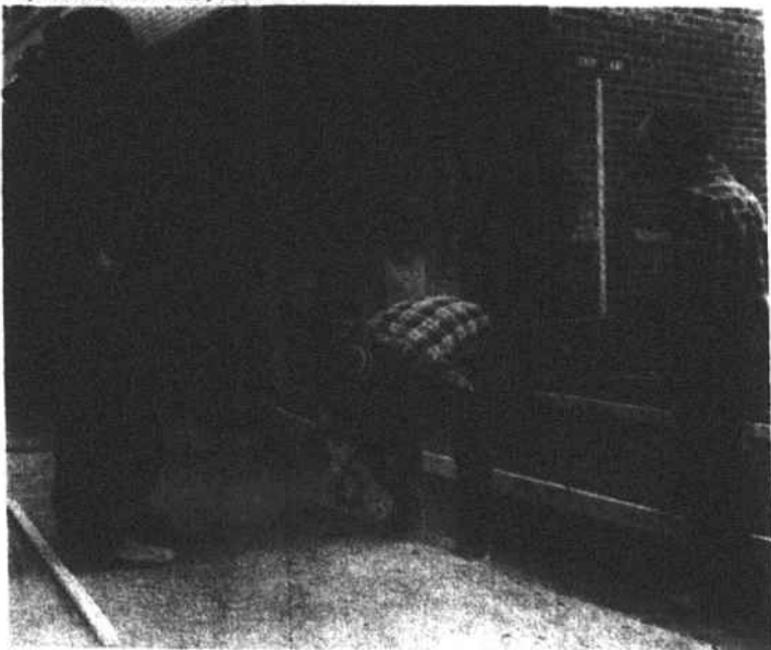
REPAIR -- Workers are giving Lundy Lane at West Elwood Avenue a proper entrance and exit. The state of the entry-exit has been a source of annoyance to drivers and a threat to the well being of the underworks of vehicles using it.
