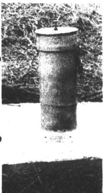
State 79-foot-deep monitor well. Note the lock to guard the interior mechanism.
