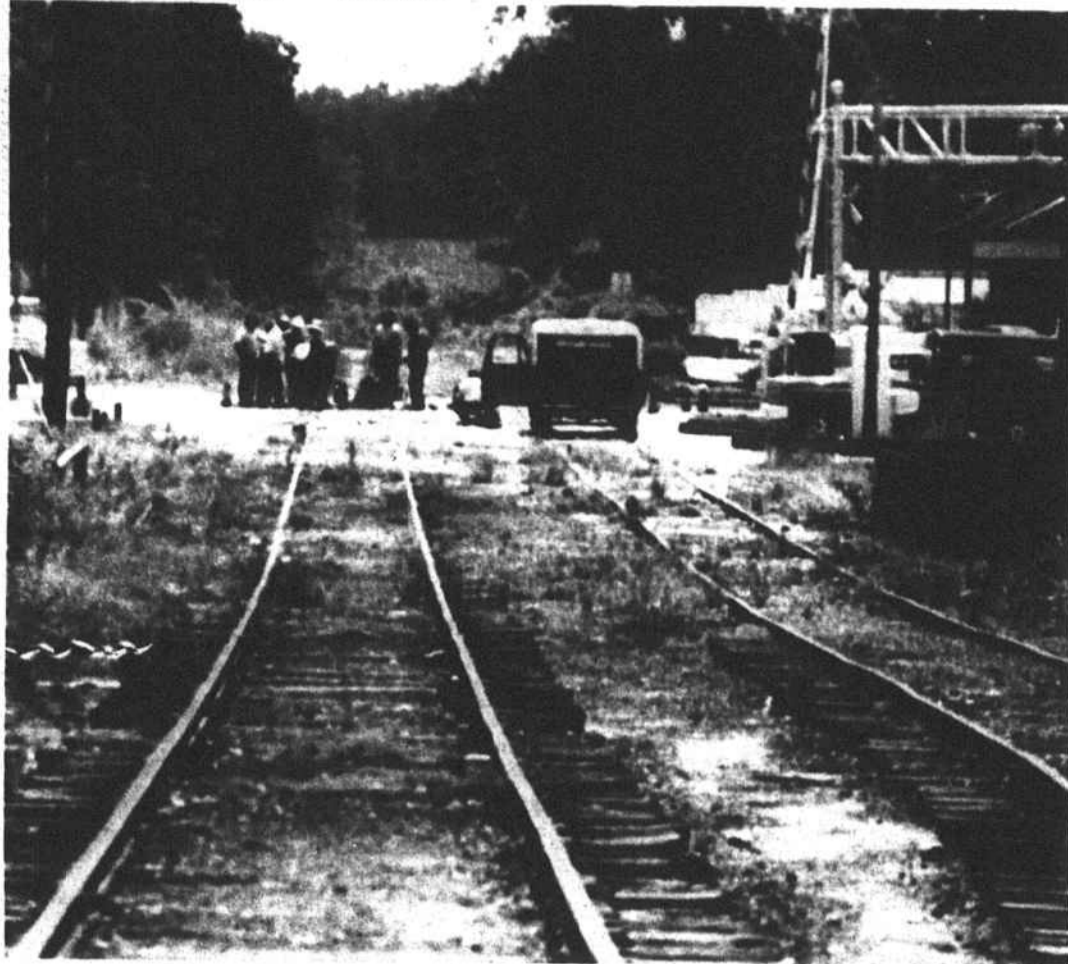
Spending time on the tracks Work crews fell into step at the railroad tracks on Main Street Tuesday to begin repairing rough railroad crossings that have been drawing complaints from city residents. At the July City Council meeting, City Manager Ron Matthews informed the members that representatives from the Aberdeen and Rockfish Railroad met with city engineers and the crossings would be repaired within 30 days. True to their word, crew members were beginning work on replacing the timbers Tuesday.
