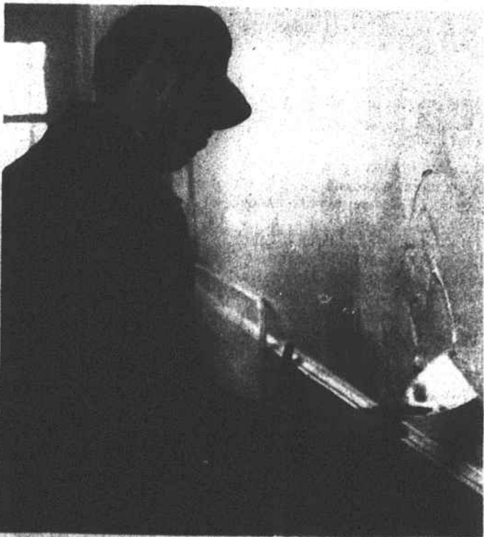
Plaster repairs Jimmy Jacobs makes a needed plaster repair in the Turlington hallway.
