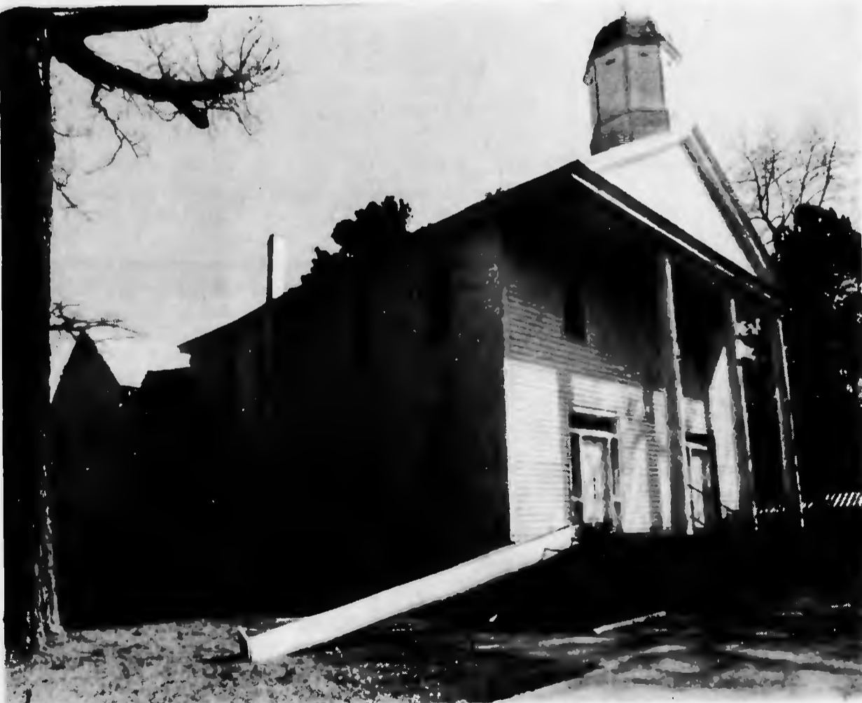
Bethel Presbyterians found this wind damage to their church from Saturday's storm. Members said it appears this column was made from a single tree. Rotten inside, it couldn't withstand 50 m.p.h. winds.
