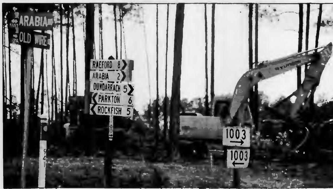
Huge trucks and all types of other equipment were hard at work last week clearing the land for the new elementary school in the eastern part of the county. The next step in the process will include awarding construction contracts for the project.
