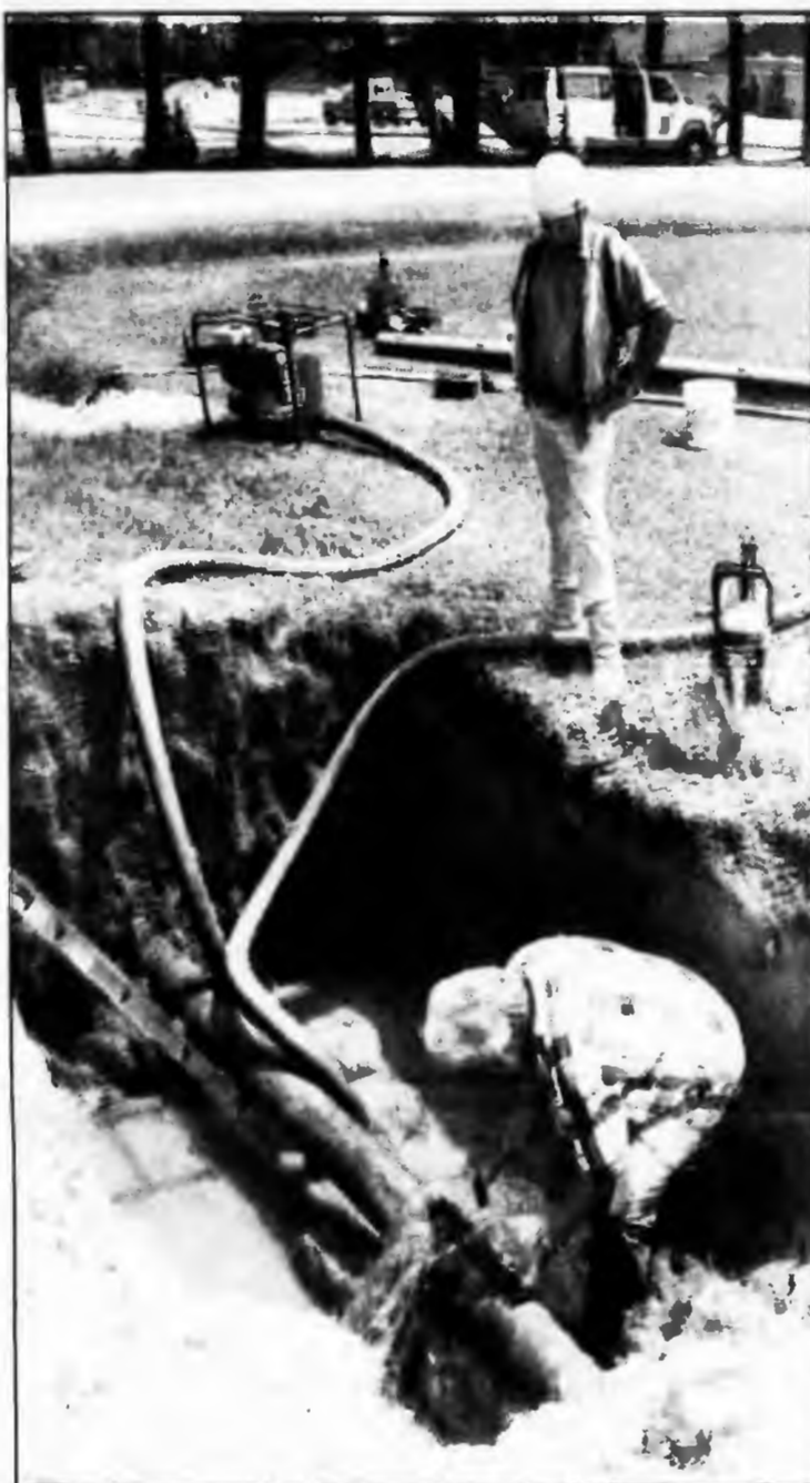
A water main is moved to make way for a new parking lot.
