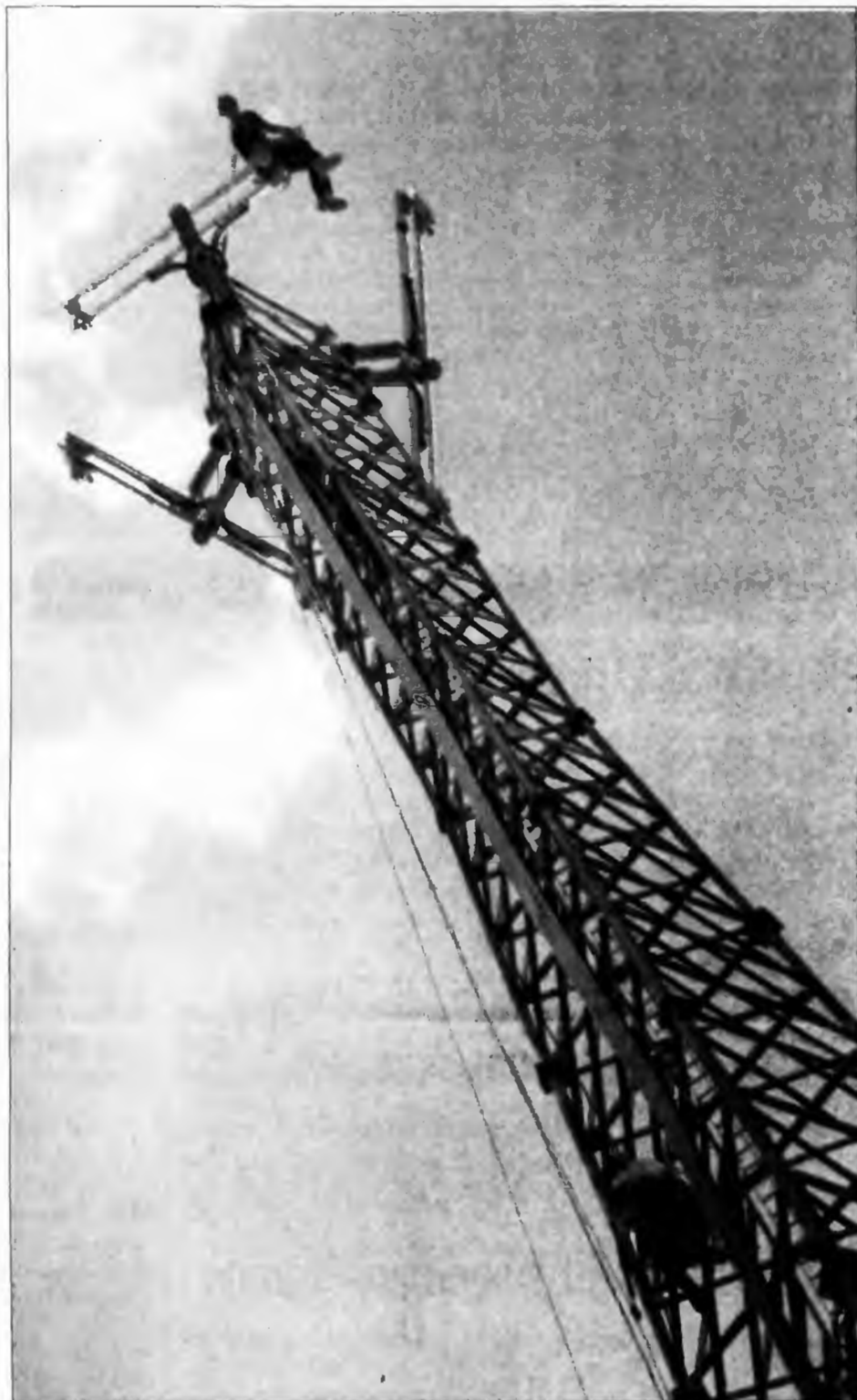
Tony Strenke, Neil Hobbs and Bryan Rose of Raleigh-based Specialty Construction Company worked on the 250-ft. American Tower Corporation structure on Aberdeen Road last week. The men were at the site Saturday morning braving winds from a menacing Dennis.
