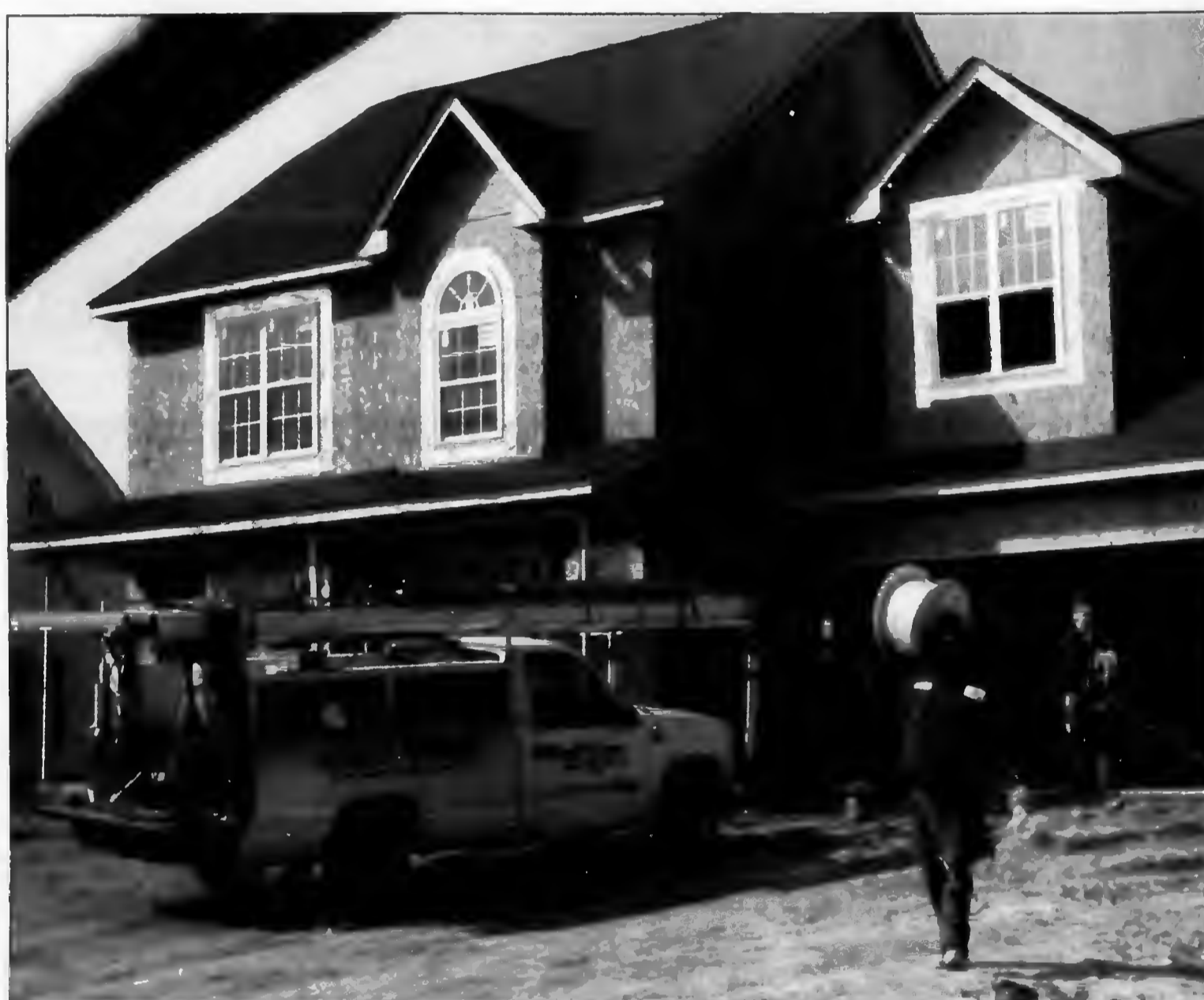
A home in the Hollies at West Gate is constructed using a panelized technique which enables builders to complete a home in nine days.
