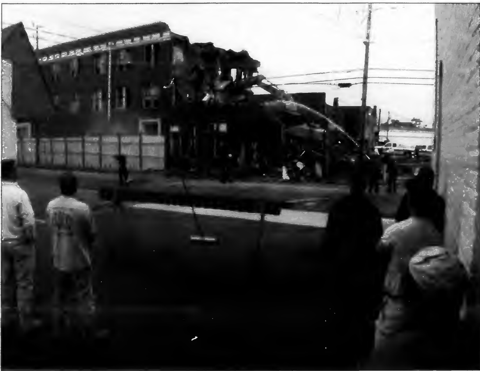
Going ... going ... The old Raeford Hotel falls to a demolition crew Friday as bystanders look on. By the end of the day, the building was just a pile of rubble.
