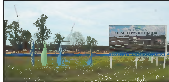
Cranes raise steel, and a sign shows what the buildings will look like at the Cape Fear Valley site on US401.
