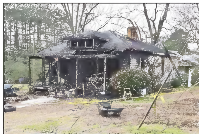
This South Stewart St. house is a total loss. (MacDonald photo)
