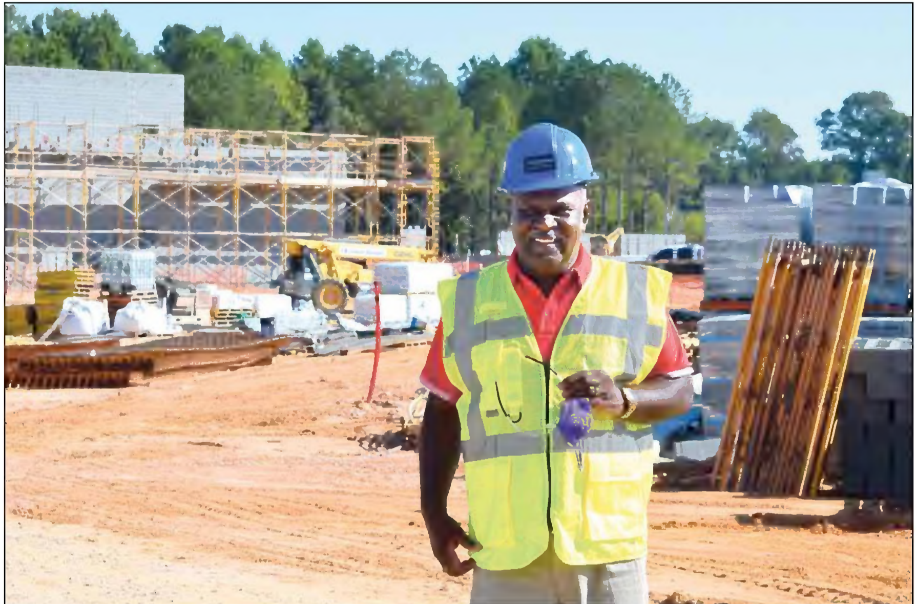
Hoke Commissioner James Leach, the man for whom the aquatic center is named, shows construction progress Tuesday. (Catharin Shepard photo)
