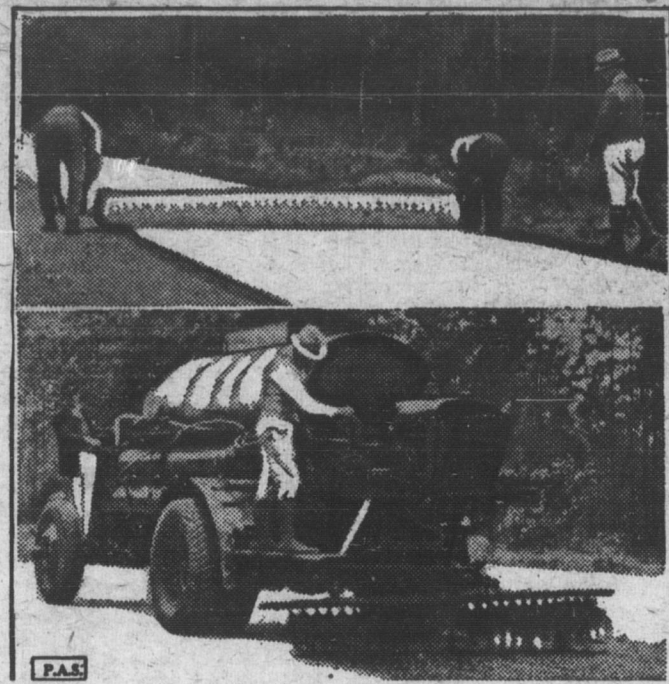
SCOTT, Mis. . . The first "Cotton Highway", a 14-mile experiment in road construction, is rapidly nearing completion here. The upper picture shows the cotton fabric membrane being rolled out on the highway on a base of mixed clay and gravel. Lower picture shows coat of far over cotton, this covered with two applications of asphalt mixed with screen gravel.
