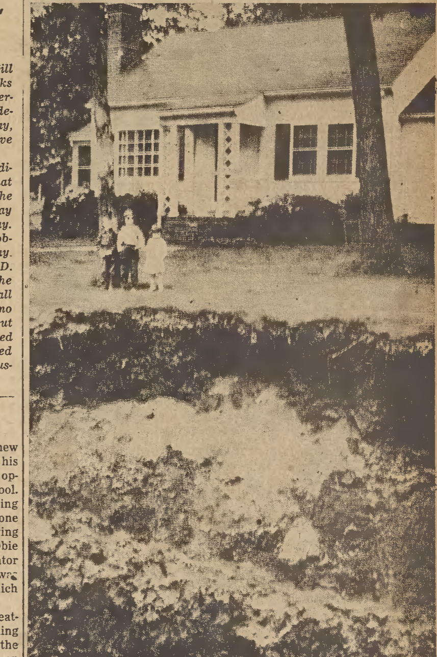
FRONT YARD BOOBY TRAP —Max Saunders and his family on Oakwood Drive looked out on a 20-foot chasm in front of his house for several months recently during the agonizing process of having a sewer line installed on the street. Above, children peer over the brink of the unguarded hole. The job is almost finished now, almost eight months past the original contract date. News Leader Photo
