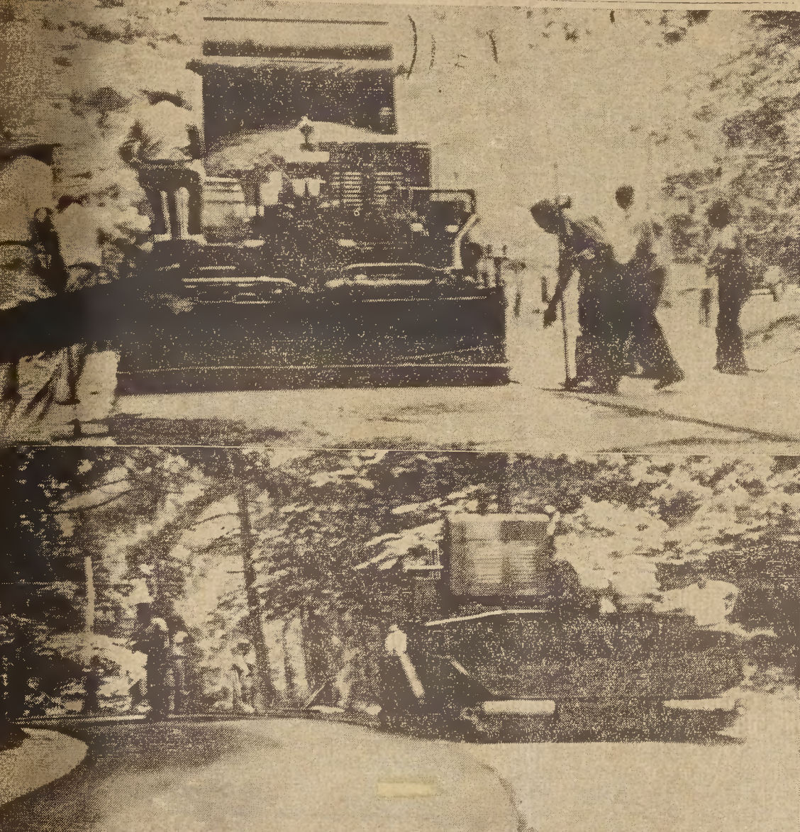
PAVING UNDERWAY —Residents of Westwood and Forest Hills, accustomed to mud-ruffed roads for many years, watched with delight this week as workmen and machinery of the William Reed Construction Company of Durham laid down a plant-mix black-top surface on their streets. The paving machine, shown in action above on Dogwood Drive, moved along at the rate of several minutes as trucks dumped their six-ton loads of black-top mixture into the hopper. Each load produced a 10-foot wide paving strip, approximately 85 feet long. The nominee for the most unpleasant job of the season is the man who drives the machine, shown above sitting on his perch directly over the hot plant mix. It has to be laid at a temperature of about 300 degrees. Add this to the 90-100 degree weather we've been having and you'd swap jobs with him. The paving program will probably next week into the Stroud Hill area and later to the Roberson-Graham Street area. Patching work will be done after the regular paving is completed.
