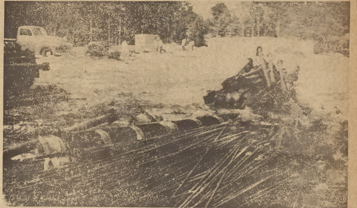
TV TOWER-TO-BE —The hundreds of assorted cross-beams, girders, poles, and wires that will soon be the 750-foot transmitter tower of Station WUNC-TV lie on the ground at the transmitter site on Terrell's Mountain in Chatham County eight miles southwest of town. In the background, looking in the direction of Chapel Hill, may be seen the work crew of the William Muirhead Construction Company which is building the transmitter building. Work on erection of the tower will begin tomorrow.
