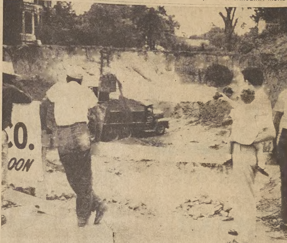
BEST SHOW ON MAIN STREET —A continuing feature that keeps getting better as the hole grows deeper, the excavation work at the Bell-Leggett site on West Franklin Street is the best show on Main street for hundreds of sidewalk superintendents each day. Young and old folks alike delight in leaning on the single-plank fence to watch the big power shovel scoop up truckload after truckload of earth. The hole will be all scooped out soon and construction of the branch of the Durham department store will begin. —News Leader Photo
